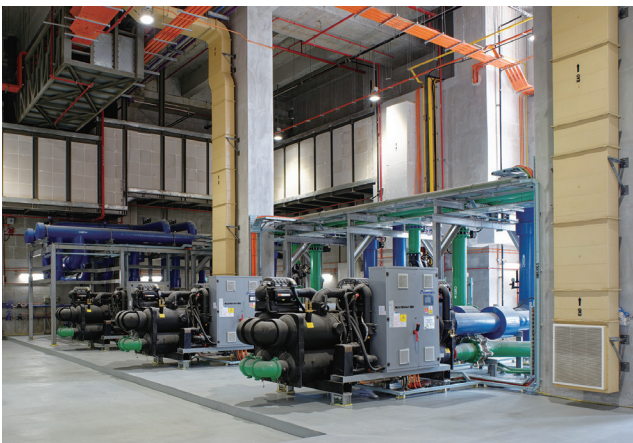
Chiller Plant Room
