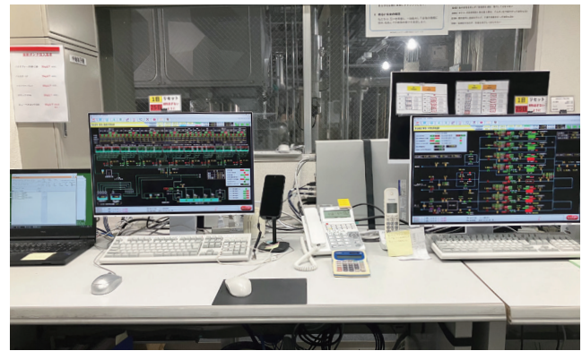
Central monitoring equipment of No.1 Plant
