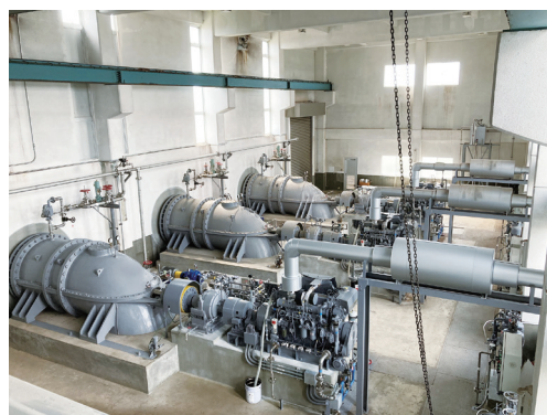
Daifu River Drainage Pump Station after the maintenance and renewal of mechanical facilities
