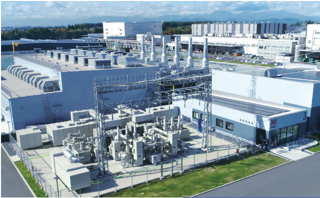
Kiyohara Smart Energy Center (Utsunomiya City, Tochigi Prefecture)
