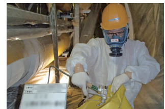
Spray and Disposal of an Agent to Prevent the Scattering of Asbestos
