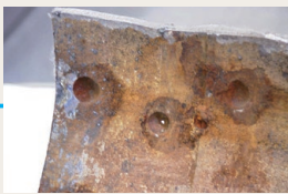
Signs of corrosion like locally stripped circles
