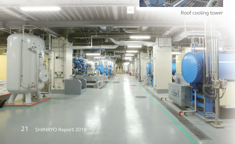
Basement machine room
