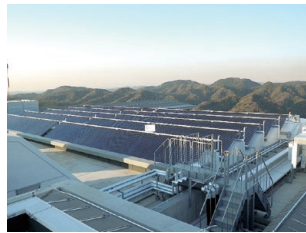
Solar hot water supply systems
