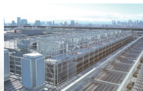
Roof cooling tower
