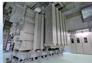
Extra-high transformer (77 kV/6.6 kV 10 MVA)
