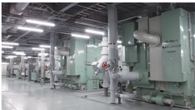
Heat Source Machine Room
