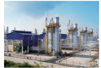
Petronas Penapisan (Melaka) Sdn Bhd Cogeneration Plant Plant facilities (Malaysia)
