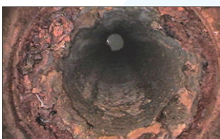
Without introduction of the corrosion prevention system
