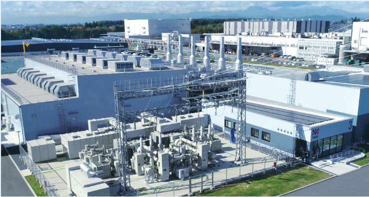
Kiyohara Smart Energy Center (Utsunomiya City, Tochigi Prefecture)
