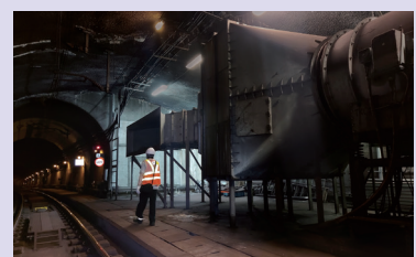
Ventilation fan in the subway tunnel
