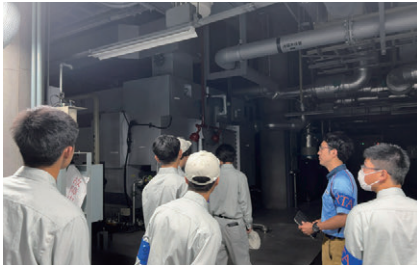
Heat source machine room tour
