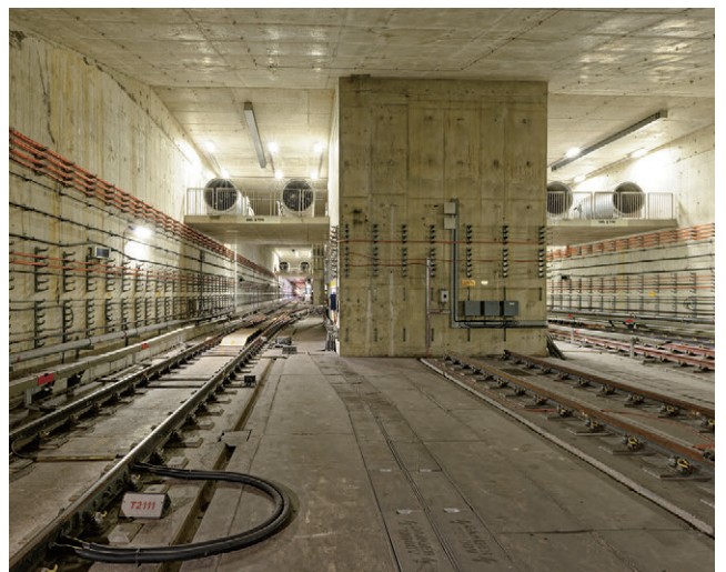
Tunnel ventilation system
