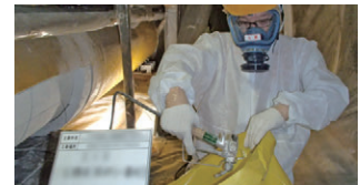
Spray and Disposal of an Agent to Prevent the Scattering of Asbestos
