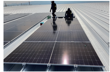
Photovoltaic generation system
