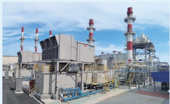
GSPP Cogeneration Plant (Malaysia)
