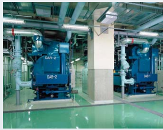
Nishi Shinjuku 6-chome Area DHC facilities 3rd Plant DHC (Shinjuku-ku, Tokyo)
