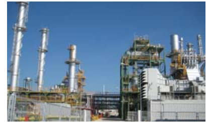
PTT Utility Co. Ltd. Central Utility Plant 2 (Thailand)
