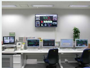
Kinshicho Heat Supply Central Monitoring System (Sumida-ku, Tokyo)
